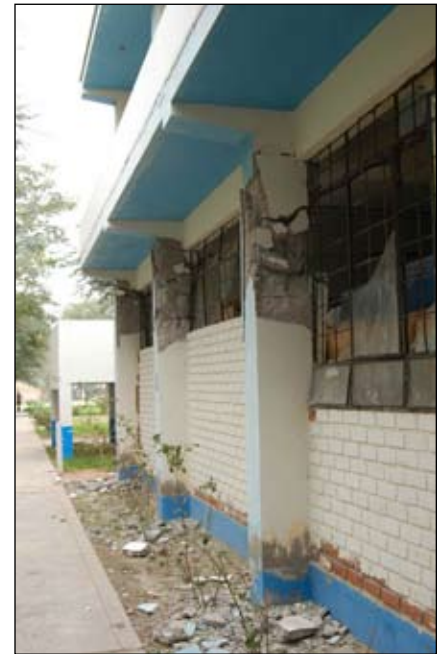
Figure 16. Damaged building at the University San Luis Gonzaga due to short columns.
