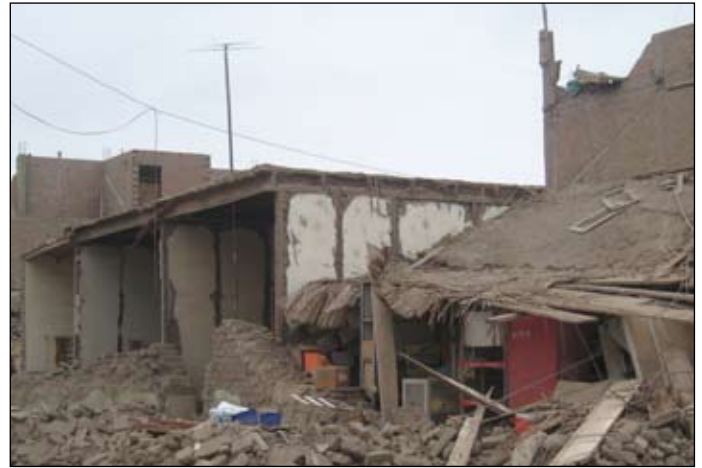
Figure 10. Two collapsed adobe houses in Pisco. The roof joists of the house on the left are supported on the quincha partitions. The roof joists of the house on the right were supported on the façade wall, and thus collapsed with the façade. Notice the undamaged confined masonry house at far left.
