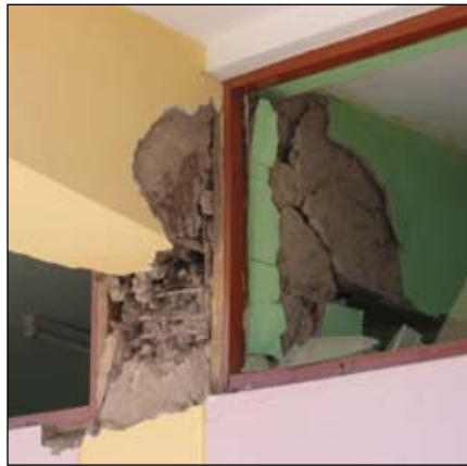
Figure 15. Shear failure of short columns next to corridor.
