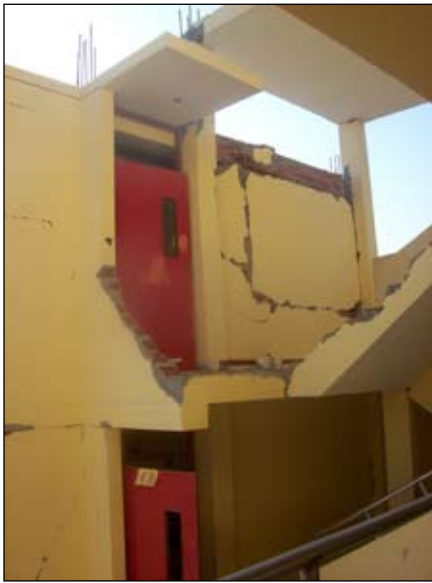
Figure 14. Extensive masonry wall damage.
