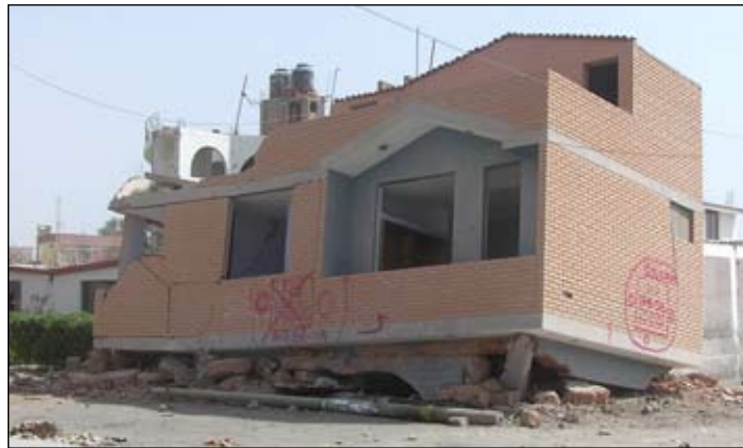
Figure 13. Confined masonry with soft stories, relevant irregularities, or bad detailing, collapsed or showed severe damage.
