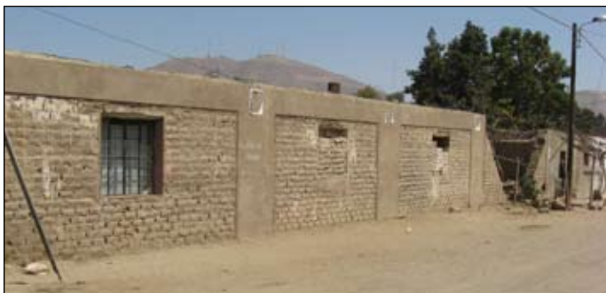
Figure 11. This undamaged adobe house was reinforced with bands of wire mesh covered with sand-cement mortar. Vertical bands were placed at each wall intersection, and horizontal bands at roof level. Notice the collapsed unreinforced wall at the right.
