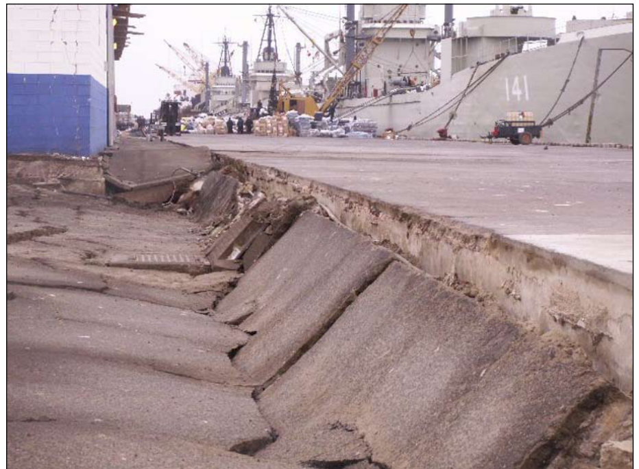
Figure 21. The fill behind a sea wall settled about 1 m at the Terminal Marítimo General San Martín.
