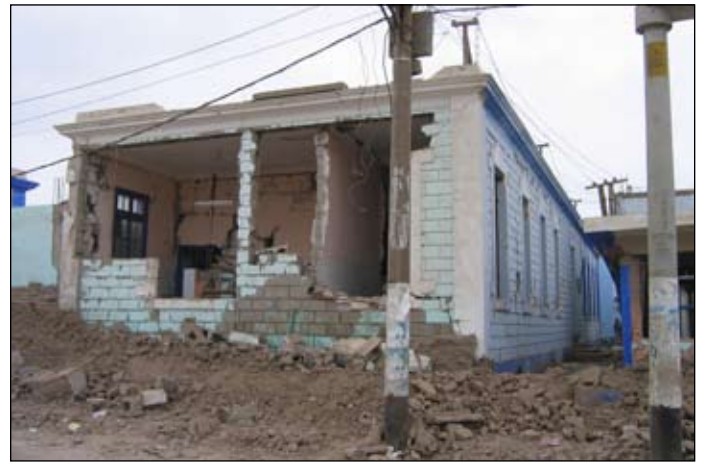
Figure 18. Damage to a Pisco Hospital building with window openings at one end and a door opening at the other.
