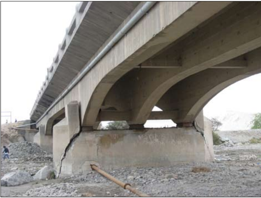
Figure 20. Evidence of liquefaction was observed at three piers of the Huamani Bridge along the Pan American Highway and in the surrounding area.
