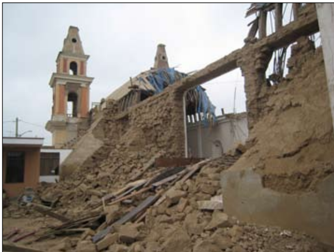
Figure 12. San Luis Church. The lateral wall and its heavy abutments were torn down, presumably by the dynamic thrust of the collapsing vault.
