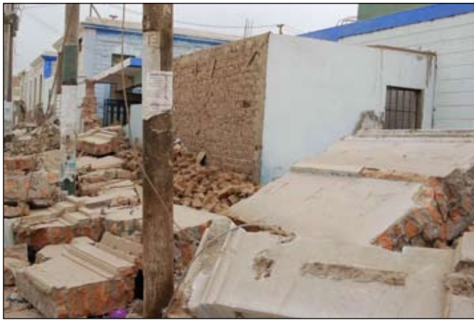
Figure 17. Damage to Pisco Hospital.
