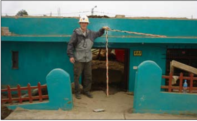
Figure 5. Approximately 0.9 m of liquefaction-induced settlement at a one-story residence in Tambo de Mora.
