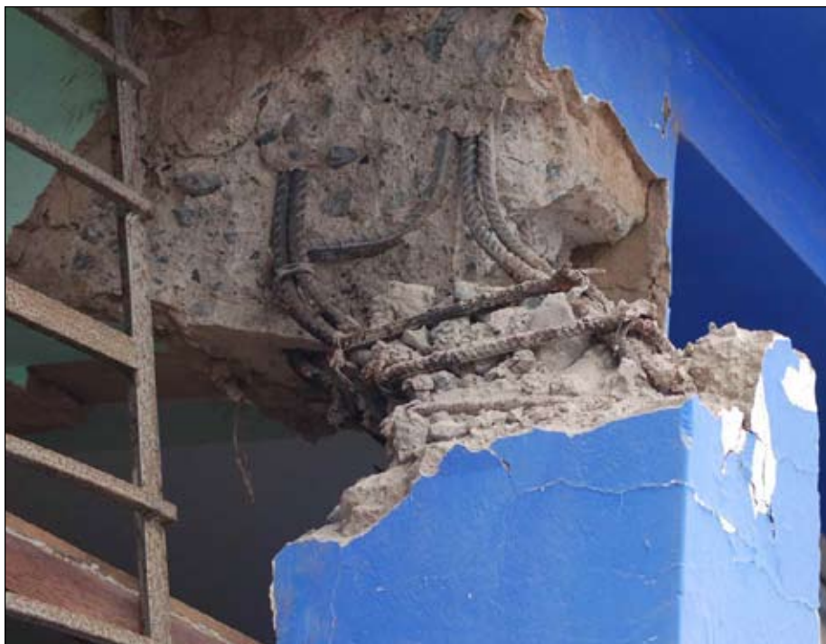
Figure 19. Damage to a reinforced concrete building at Pisco Hospital.
