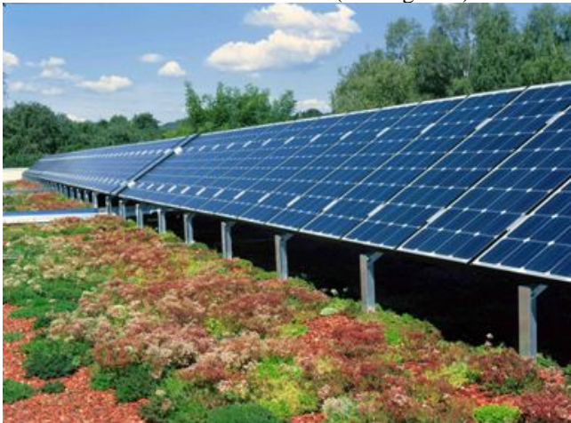
Figure 9 - Unterensingen, Germany; Primary and Secondary School extensive green roof with photovoltaics ( www.greenroofs.com/projects , accessed 7/4/08)
