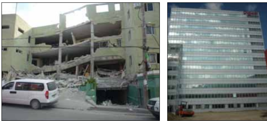
Figure 6. Differential damage to two structures across the street from one another in Port-au-Prince: (a) reinforced concrete frame with masonry infill; (b) new Digicel building under construction
