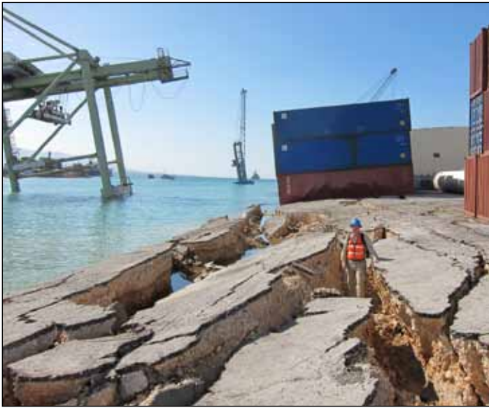
Figure 9. Fissures caused by lateral spreading at western ends of the North Wharf.
