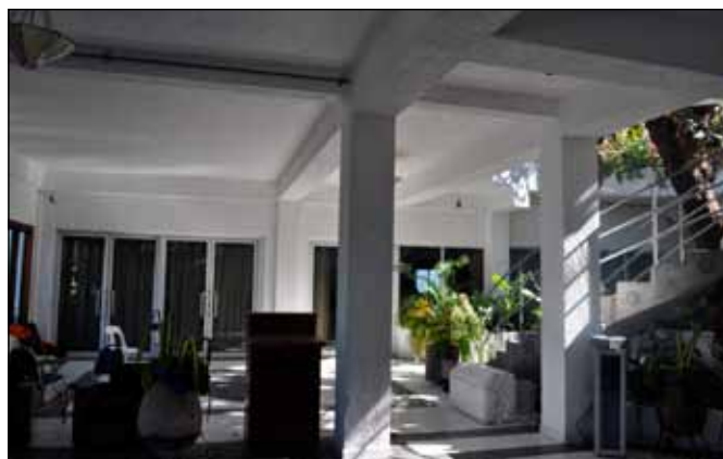
Figure 8. Areas of the Hotel Montana lobby remained intact. It appeared that this part of the building had reinforced concrete beams and slabs without extensive infill walls.
