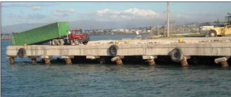
Figure 11. Remaining portion of pile-supported pier at the Varreux Terminal (source: Chodkiewicz).
