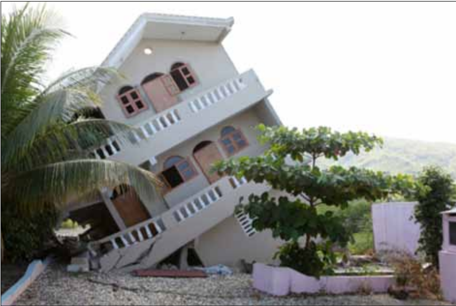
Figure 3. Combined structural and foundation failure southwest of Léogâne.
