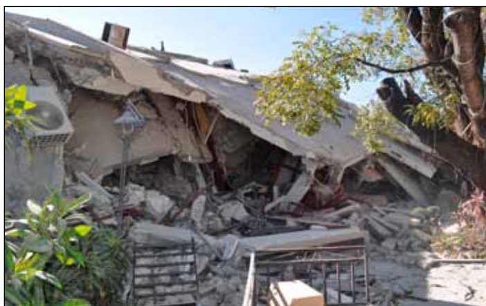
Figure 7. Collapse was extensive throughout the guest wings of the Hotel Montana, constructed of reinforced concrete with unreinforced infill concrete masonry walls.
