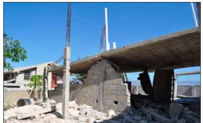
Figure 5. Partial collapse of residential building under construction.
