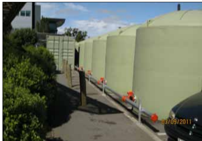
Figure 20. Temporary water tanks in front of Christchurch Hospital (photo: Gavin).
