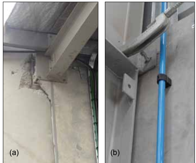
Figure 14. Damage to industrial buildings at steel-to-concrete connections: a) roof beam-panel connection in load-bearing tilt-up building; b) steel frame-panel connection in building with nonload-bearing concrete panels (photo: Marshall).
