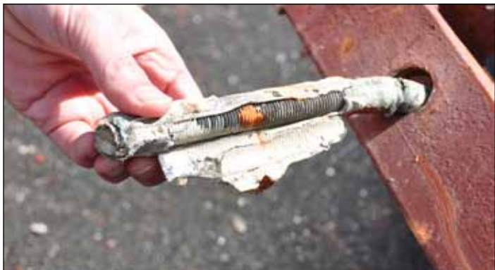
Figure 16. This adhesive anchor at a URM parapet connection pulled out. A wire screen with white adhesive around the threaded rod had been inserted into a hole in the brick (photo: Turner).
