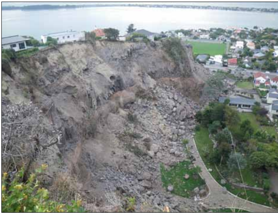
Figure 5. Large and damaging rockfall behind Moa Cave Guest house, Red-cliffs (photo: Mote).
