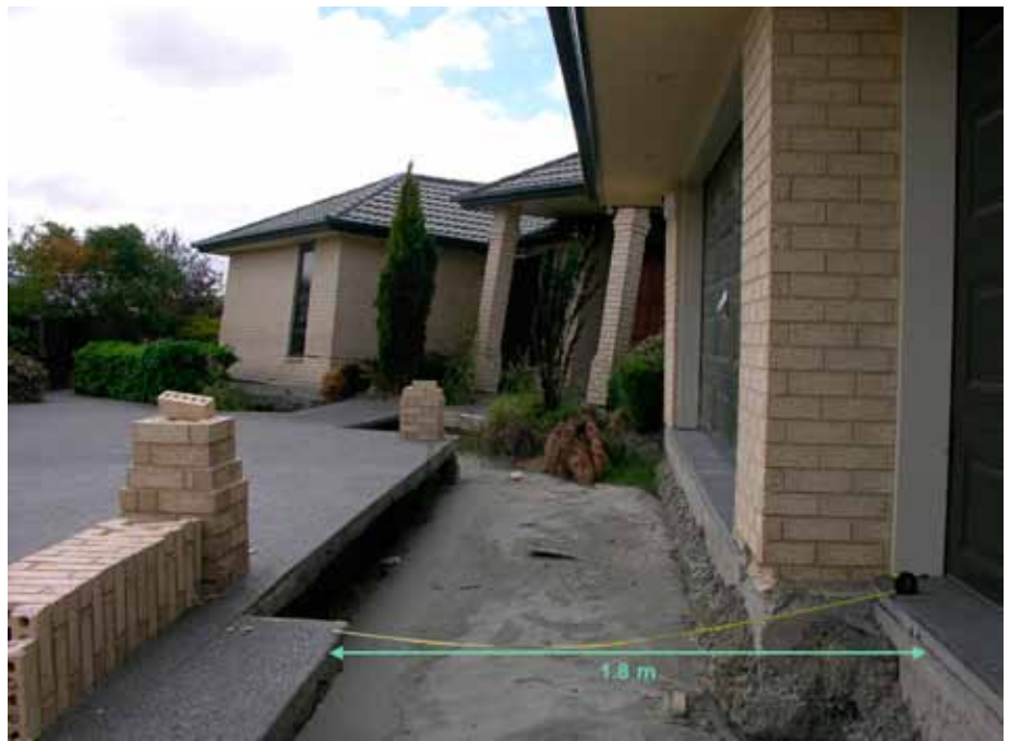
Figure 21. A house in Kaiapoi moved on its foundation in both the September and February earthquakes a total of 1.8m (photo: Lai).
