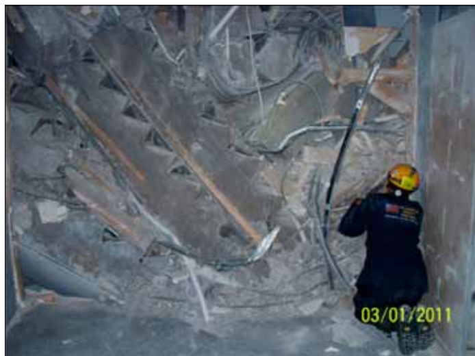
Figure 13. Collapsed precast concrete stairs in multi-story building (photo: Carri).
