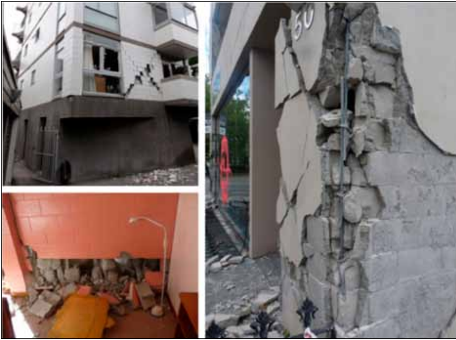
Figure 12. Examples of reinforced masonry damage in multi-story buildings (photos: Jaiswal and Sritharan).
