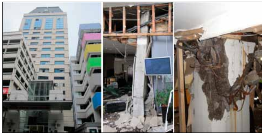
Figure 9. A permanent twist and residual lateral displacement in the 19-story Hotel Grand Chancellor (photos: Elwood, Comerio).
