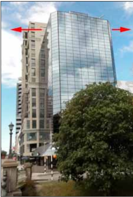
Figure 6. Differential movement of adjacent buildings (approximately 700mm at roof level) due to foundation rotation (photo: Elwood).
