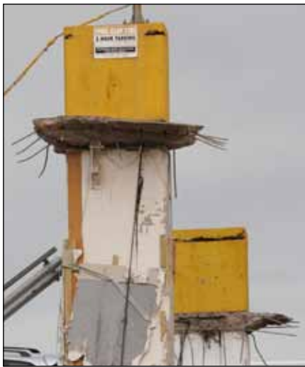
Figure 8. Punching shear failures in parking garage (photo: Berkowitz).
