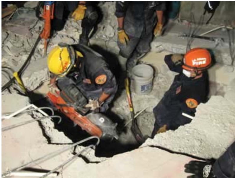
(8) Rescuers used vertical breaching to reach Makinson. Even with power tools, it was a slow, laborious, meticulous process to reach the trapped man.
